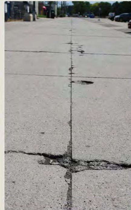
Cracked and damaged concrete along the alley
