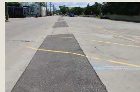
Parking slope does not meet ADA standards
