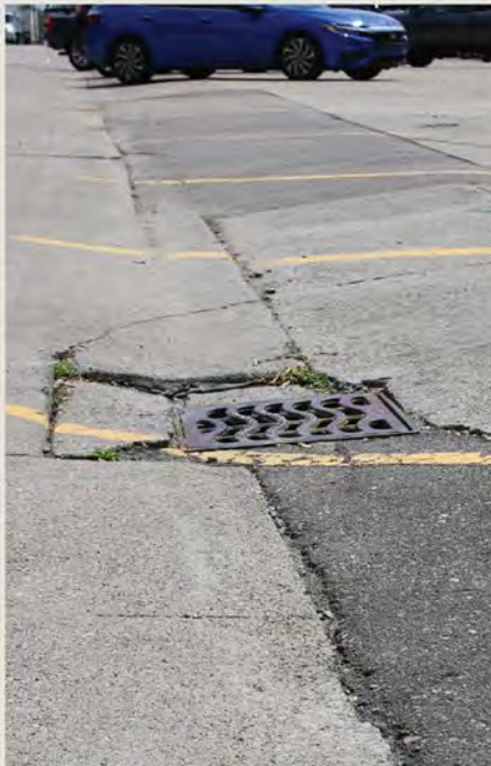
Cracked & unlevel concrete around the storm drain
