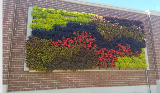
LANSING BWL - CENTRAL SUBSTATION
